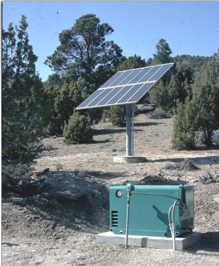
Solar panels and 4Kw propane back-up generator
